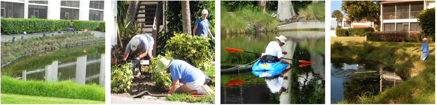
Above Geo-Tubing shoreline stabilization system with Florida Friendly landscaping plants ready for installation; Residents installing landscaping to intercept runoff; Checking pond depth by kayak; Algae removal with the amazing AquaRake.
